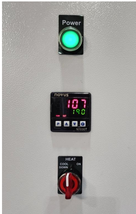
Figure 4 DRYER SHUT DOWN
